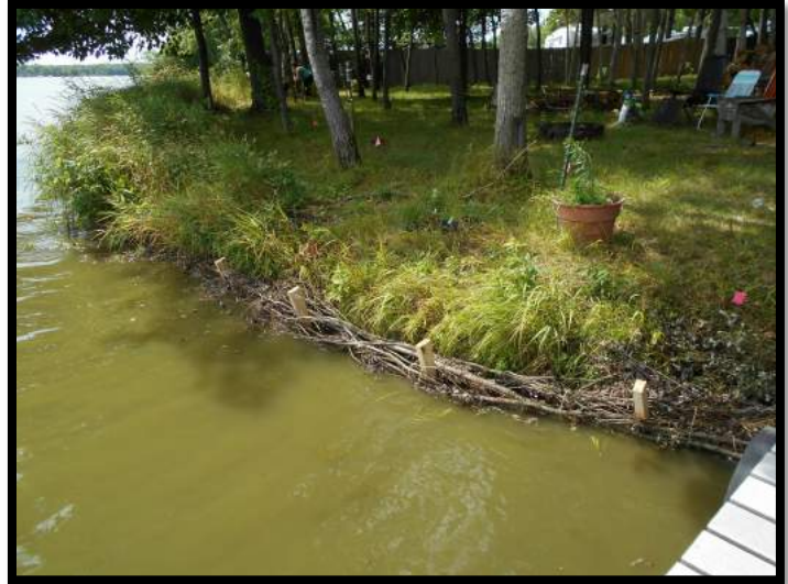
Willow wattles were used to protect the shore from erosion and to protect new plantings from wave action.
